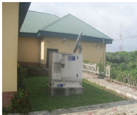
Plate 2: Vandalised Generating Set at Rumuwoji
