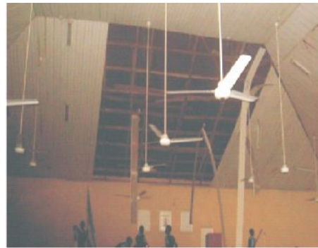
Plate 6: Collapse Ceiling in Auditorium due to Inferior Materials at Rumumasi.
