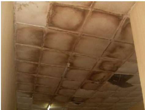
Plate 5: Rotten Ceiling in Classroom due to roof leakages at Rumueme
