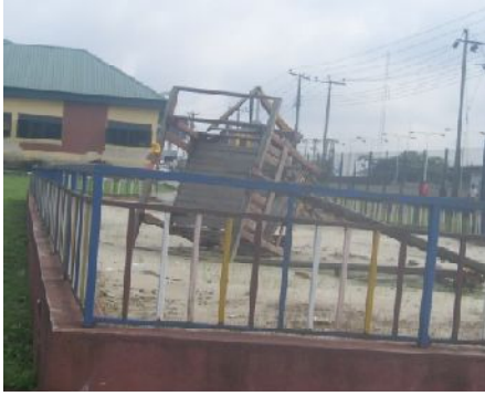
Plate 3: Damaged Recreational Facilities at Kpите
